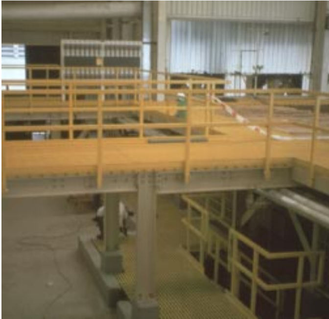
Above: Fiberglass walkways and operating platforms are used extensively in the highly corrosive SXEW copper refinery at Minera Escondida Limitada, Chile.
