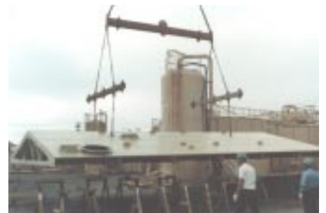
... final fabrication using EXTREN® plate and fittings was easily completed at the site.
