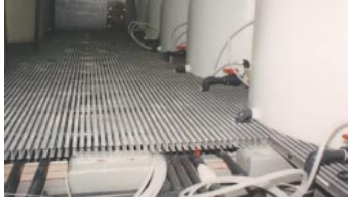
Above: A raised floor, in the processing room of a California film development laboratory, surrounds existing equipment, provides access above and below the floor, withstands the corrosive environment and provides 200 lbs/sq.ft. load capacity to support heavy machinery.
