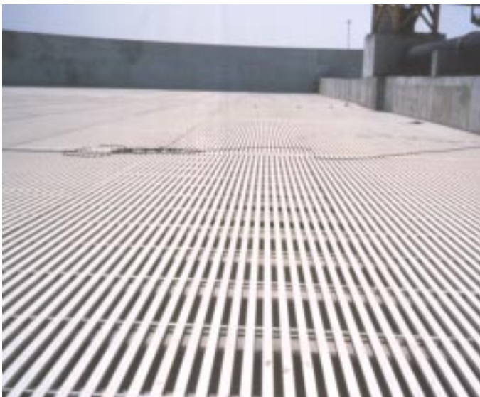
Above: Fiberglass grating was installed as media trickling filters at the Des Moines, Iowa Wastewater Treatment Plant.
