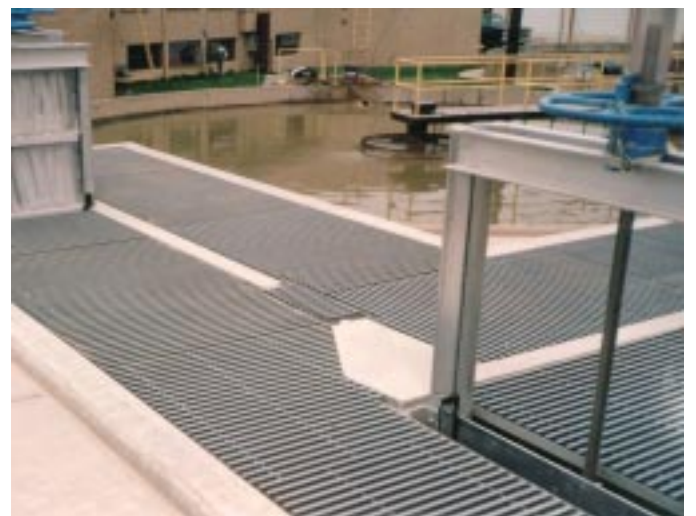
Above: Low maintenance fiberglass grating provides trouble free operations for the Wastewater Treatment Plant Headworks covers and walkways in Lakewood, Colorado.
