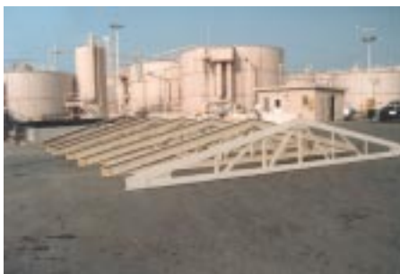
Above: Trusses for this tank cover used at a Shell Oil Refinery were preassembled and shipped to the site...
