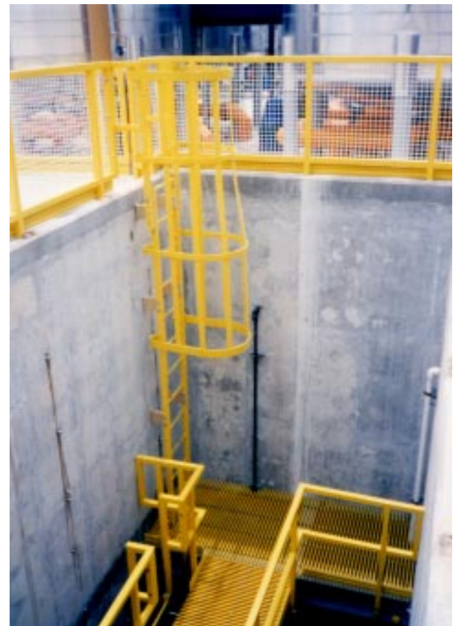
Fiberglass access ladders are used throughout the service areas of Sea World, Orlando, FL to resist saltwater corrosion and reduce maintenance costs.
