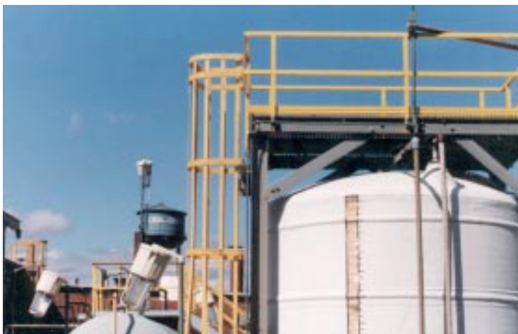
This fiberglass ladder and ladder cage provide worker access to a maintenance platform at a Ciba Geigy plant in the northeastern United States.
