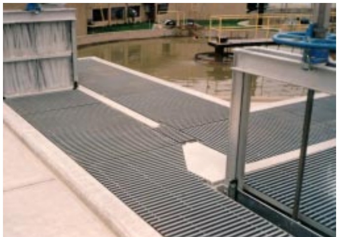
Low maintenance fiberglass grating provides trouble free operations for the covers and walkways in the Lakewood, Colorado Wastewater Treatment Plant Headworks. DURADEK® I-6000 1-1/2" was used.
