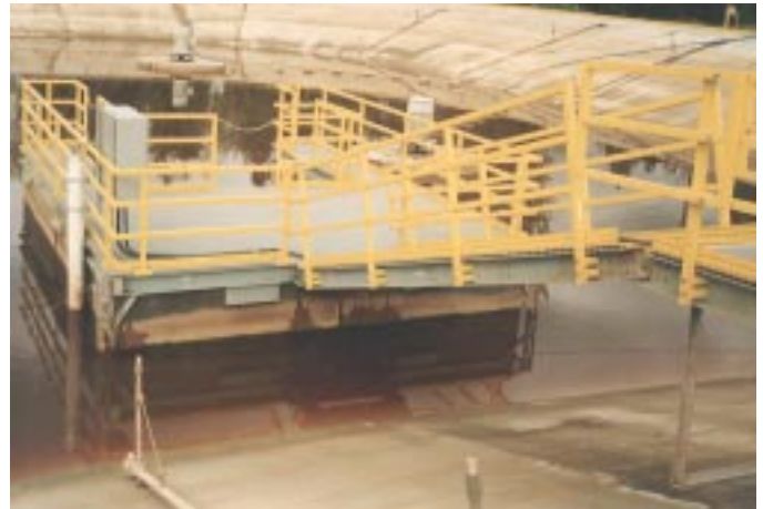
High strength EXTREN® was used to fabricate fiberglass floating docks for seepage pits at this landfill in Snohomish County, Washington.
