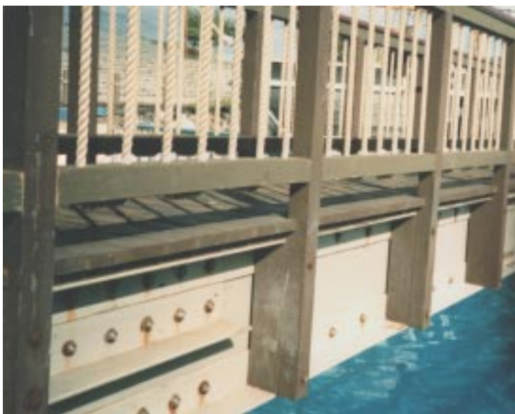
Bridges at the Sea Life Park in Waimanolo, Hawaii, use fiberglass structural supports over saltwater dolphin tanks.
