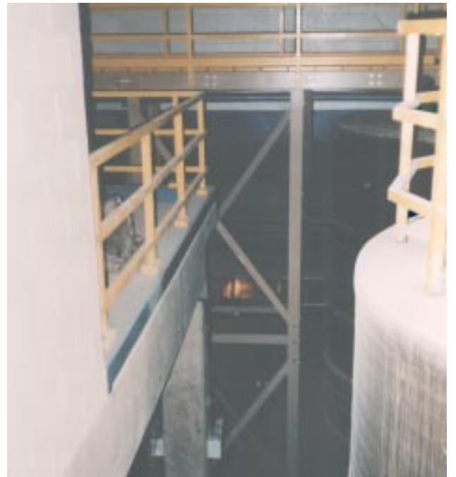
35' high platforms over tanks at Moffat Filter Plant in Denver, Colorado were constructed of EXTREN® structural shapes.
