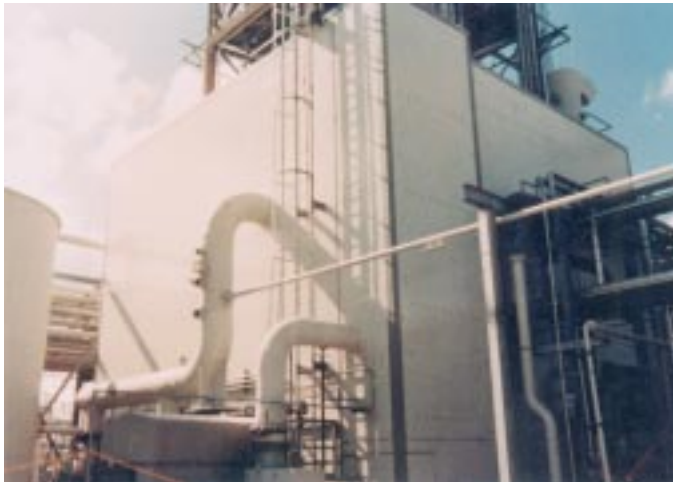
Airtight enclosure for Dow Chemical protects workers in adjacent areas against accidental escape of phosgene gas.
